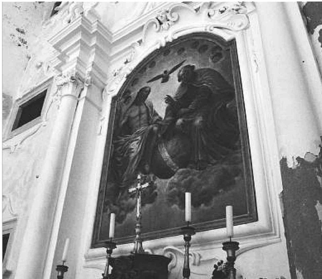
Monasteries and churches on the islands date to the 15th and 16th centuries. Some are being restored as others continue to decay.
